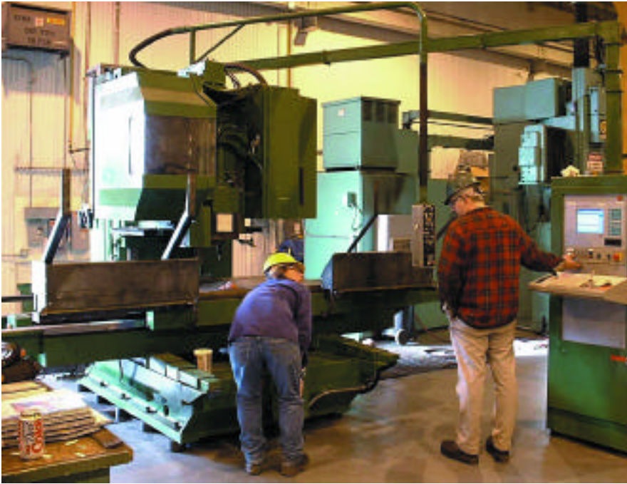
The big cabinet is almost all empty space in this Burgmaster retrofit, now that the old CNC has been stripped out. But the cabinet was already there, and the PC-based CNC fit in easily
